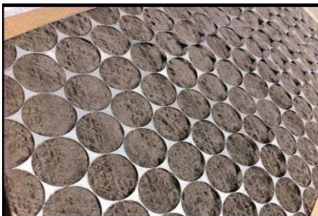
Poor Air Flow
